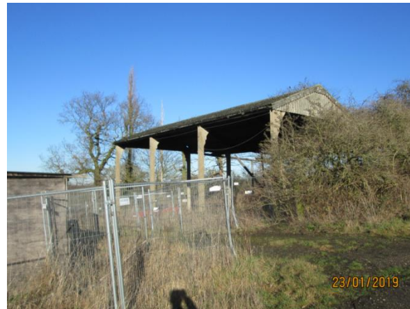
Dutch barn to be demolished. Garage for House 2 to be built in this position.
